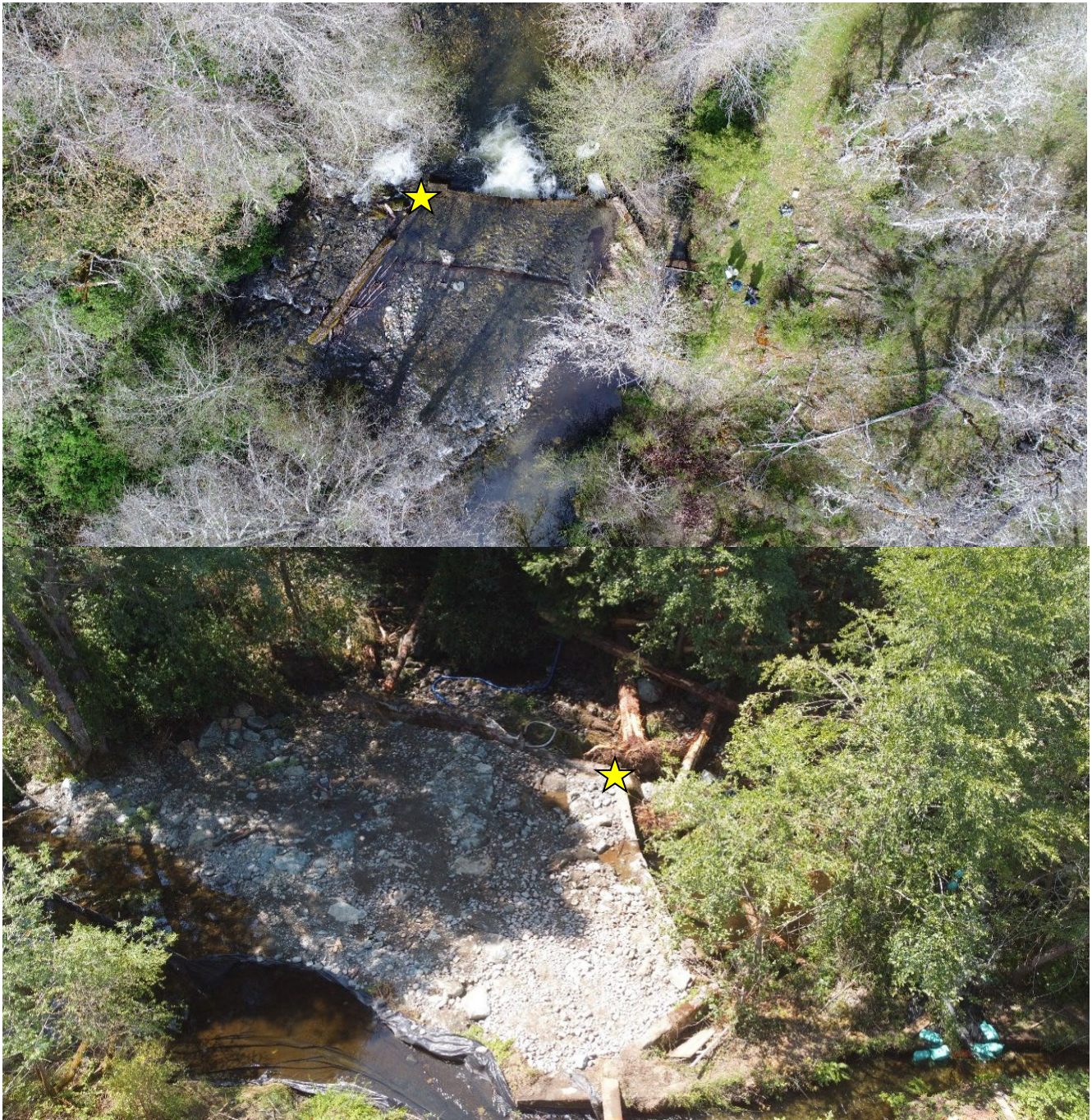
Figure 3. Aerial view of the project area at the Upper Philips diversion on Little Applegate River in Ruch, Oregon. The upper photo shows Upper Philips Dam and Ditch in 2020 before the project commenced (top). Streamflow bottom to top. The lower photo from Aug 2021 shows the completed boulder ribs/rock fill diversion structure and partial log placement in the fish passage bypass channel. Headgate/piping have not been completed in this photo and the open ditch is visible in lower right. Streamflow left to right.
