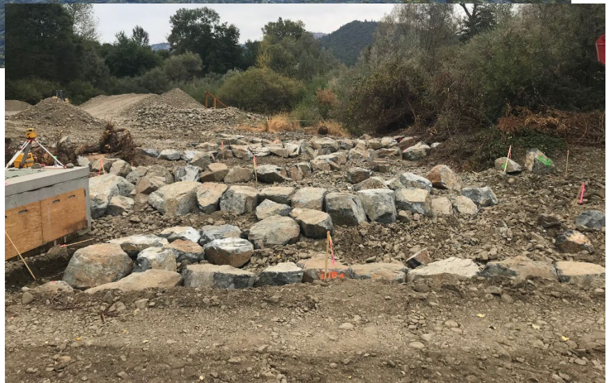
Figure 2. Looking downstream at completed Bridgepoint Ditch concrete headgate and roughened channel on Williams Creek (top). On right, same view during construction with concrete headgate and boulder ribs placed within Williams Creek channel that make up roughened channel.
